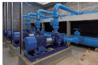
Building water pumps
